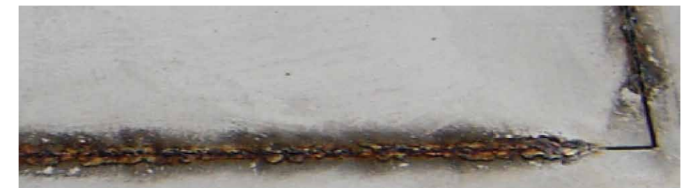
Processing defect condition (top surface)
